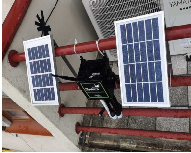
Figure 3a. Outdoor station installed on the balcony
